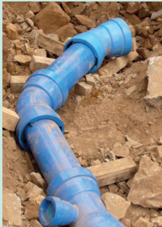
Modern installation without concrete thrust blocks
