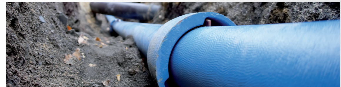
Pipeline with VRS®-T/BLS® joints as a fire-extinguishing pipeline in a tunnel
