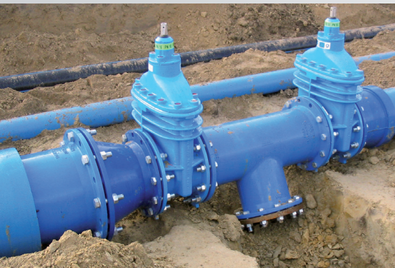
Fire-extinguishing pipeline fitted with gate valves
