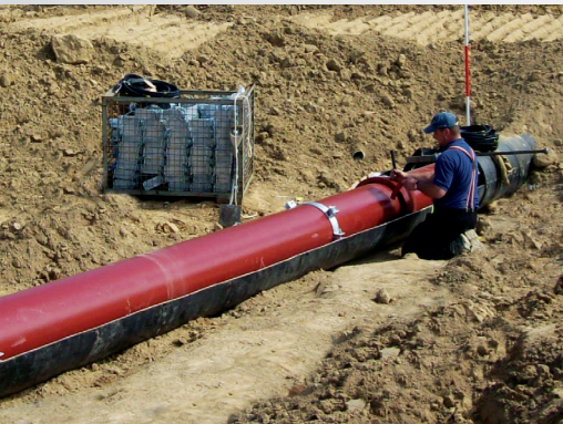
DN 400 ductile cast iron pipes with VRS®-T/BLS® socket joints being pushed into a stretch of protective tubes
